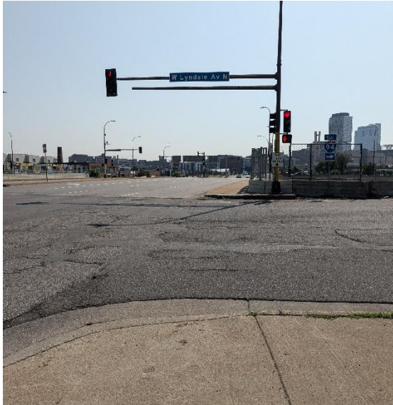
Figure 40 Missing Lane markings and pedestrian crossing.
