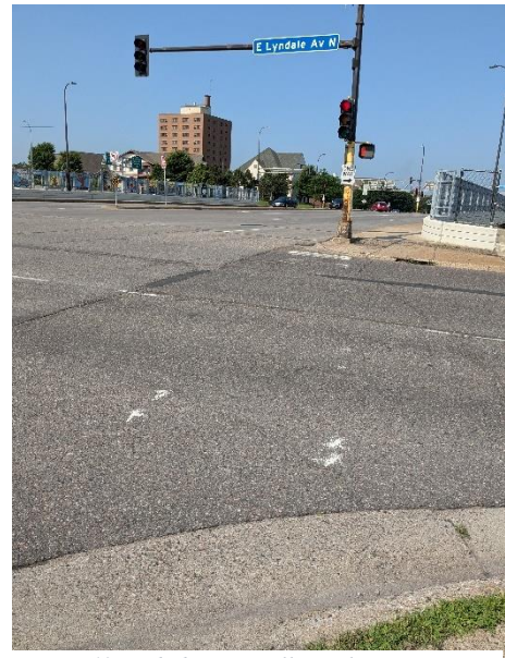
Figure 49 Faded crosswalk marking.
