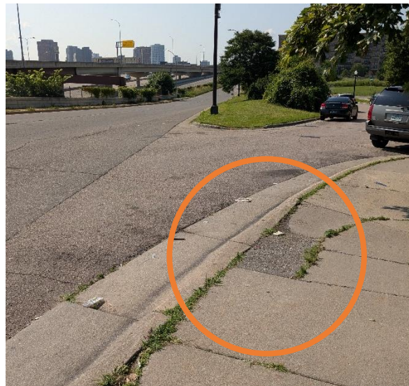
Figure 41 Curb ramp onto roadway and high-speed turn into residential area.
