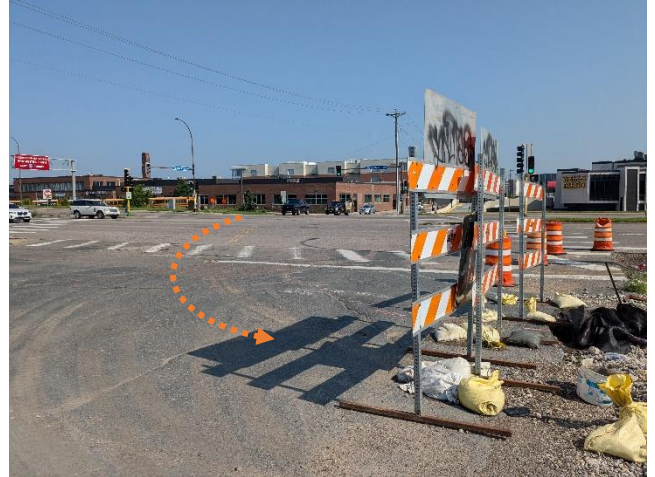
Figure 53 Incorrect yellow line extension marking.
