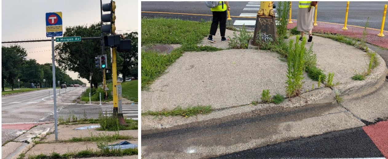
Figure 19 Poor roadway and sidewalk conditions on the corridor.
