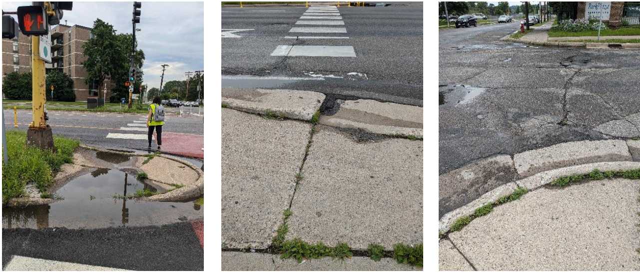
Figure 33 Pictures showing water pooling on the pedestrian crossing (left), broken pavement at curb ramp preventing access (middle), missing curb ramps (right)
