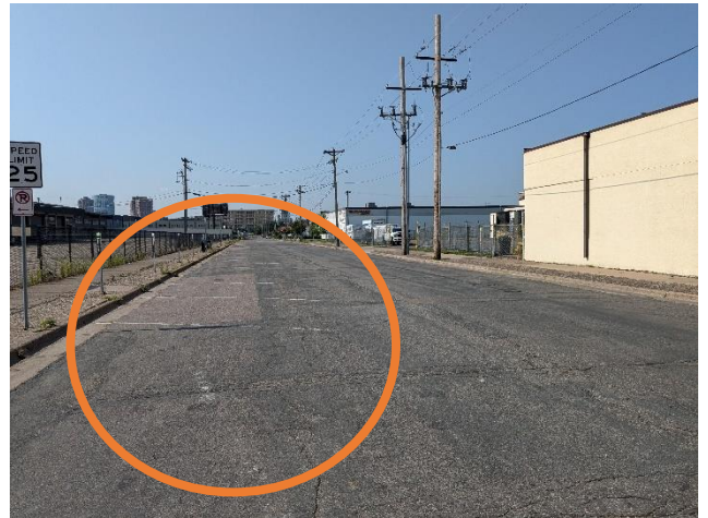
Figure 54 Faded parking and road markings.
