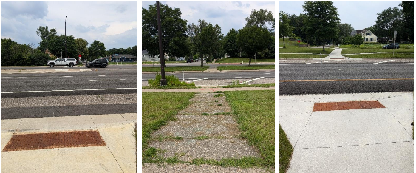
Figure 13 Examples of unmarked, mid-block crossings on Olson Hwy, including those with newer ADA-compliant ramps as well as older crossings
